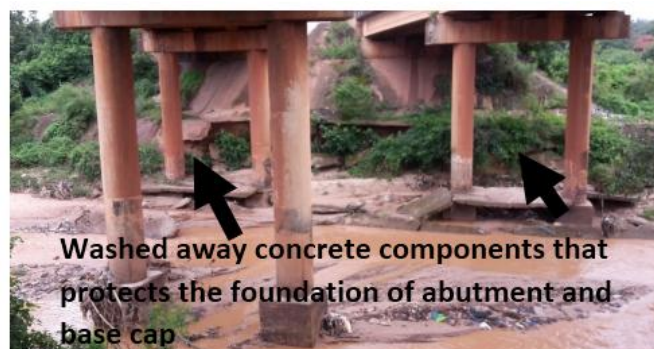
Figure 3.3 The Scouring of River-bed at Abakpa fly-over bridge
