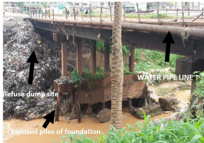
Figure 3.1 The effect of Environmental degradation on the Abakpa Bridge along Nike Road, Enugu
