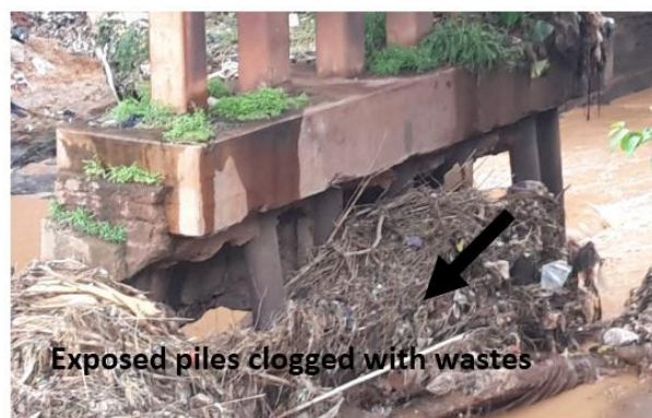
Figure 3.2 The exposed pile foundations of the center columns of the Abakpa bridge
