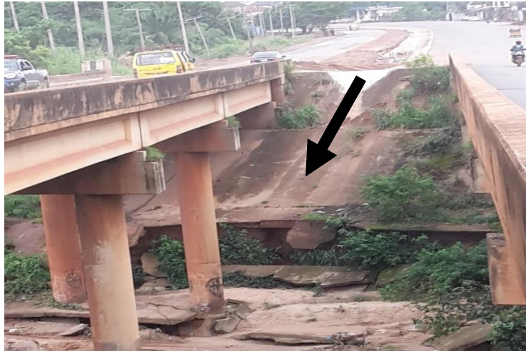
Figure 3.4 The effect of Run-off from rainfall on the concrete components protecting the abutment foundation at the Abakpa fly-over bridge.
