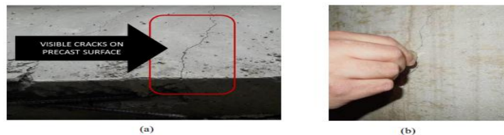
Figure1. (a) and (b) Visible cracks on Pre-cast surface.
