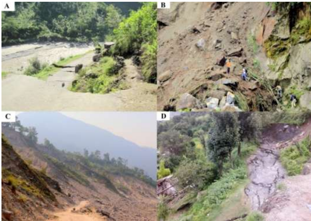
Plate-1: Impact of landslides and land creeping in district Pithoragarh: (A) Madkote to Munsyari motor road affected by land creeping (2013), (B) Tawaghat to Garbyang motor road affected by land slide (2014), (C) Ghigrani is an all-weather landslide zone (2018) and (D) Josha village affected by land creeping (2020) (based on field survey).
