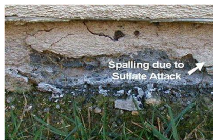
Fig 1.1.2 Spalling due to sulphate attack
